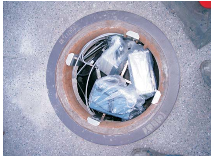
AVFM-II Electronics, Battery and RF Transmitter are installed in the manhole
