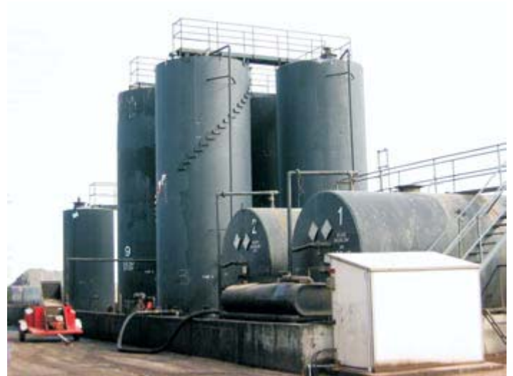
TFT32 Tank Farm Monitoring System
